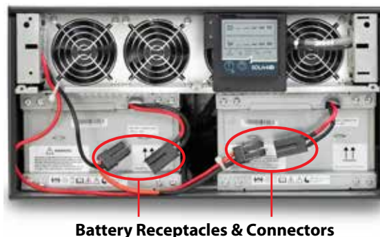
Figure 26: Disconnecting the battery packs (front view)
